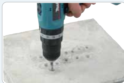
Drilled holes in Mortar with \phi 6 T.C.T. bit to a depth fo 50 mm.
